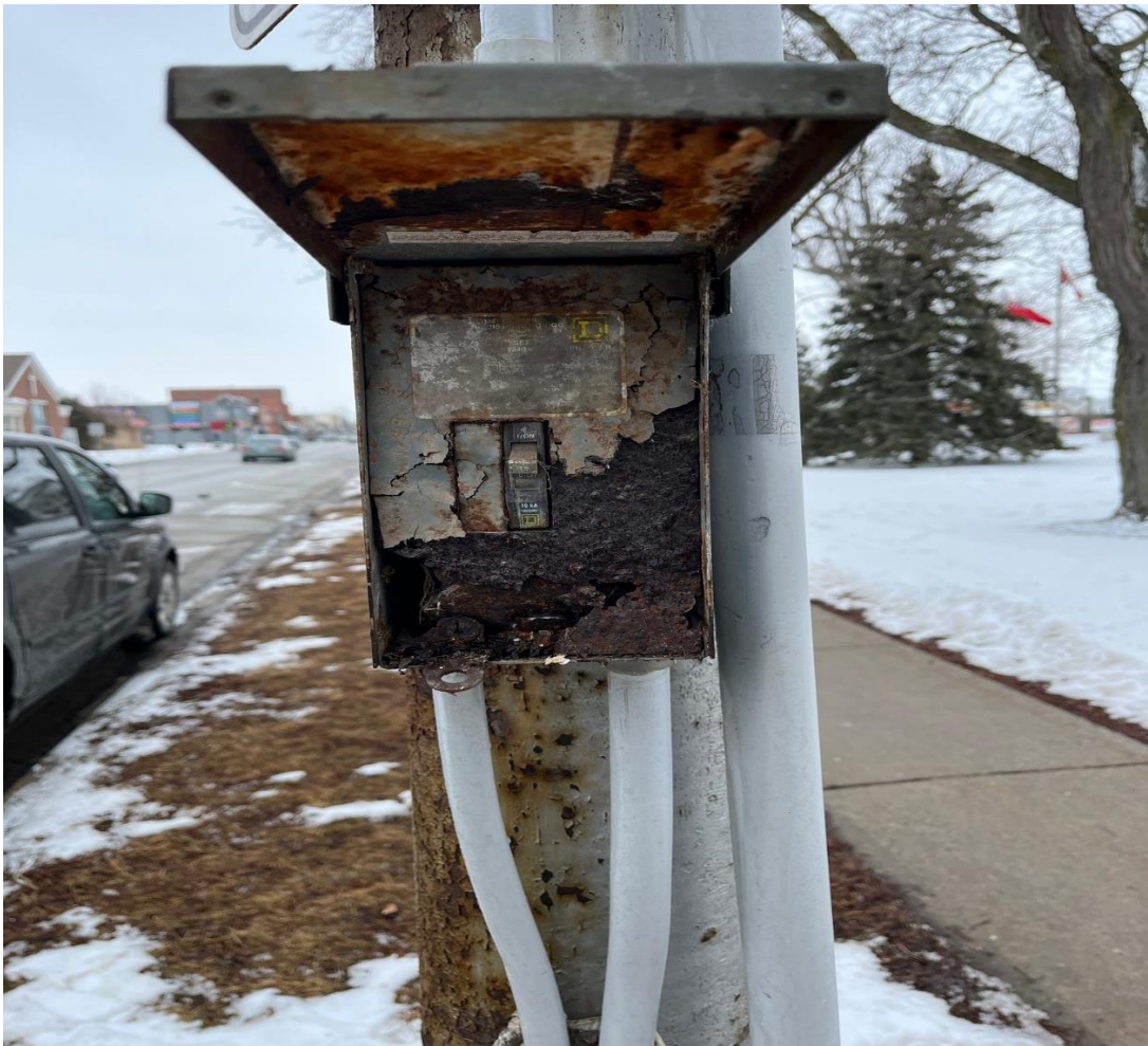
Figure 4: Essex Centre Streetlight Electrical
