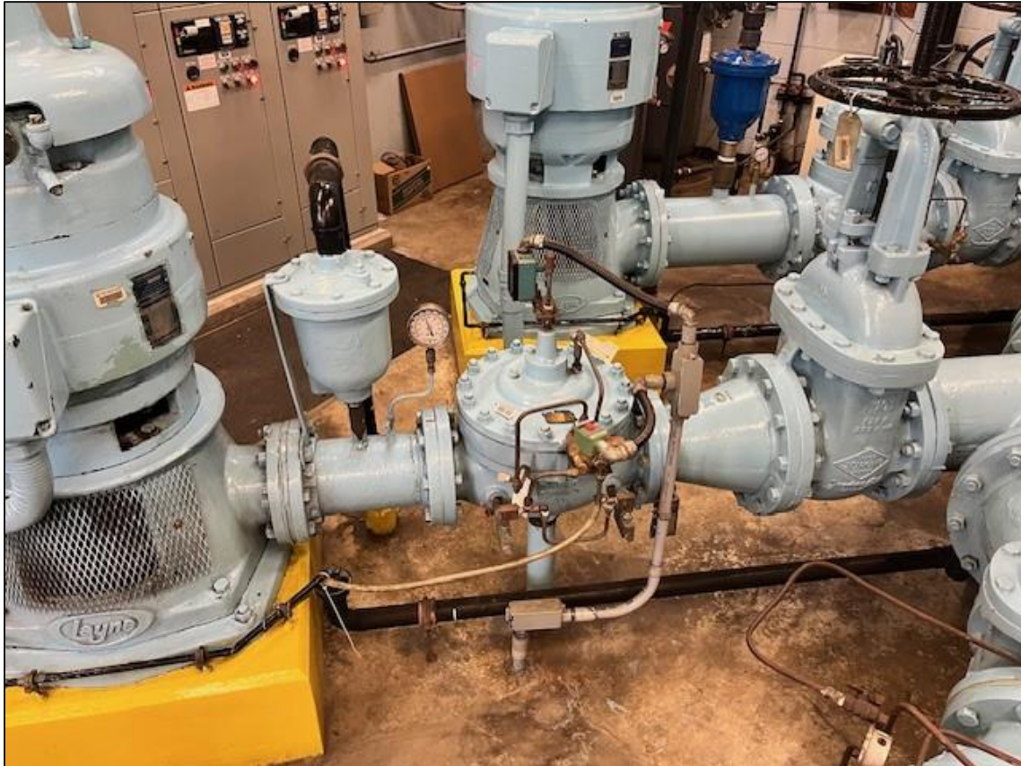
Figure 1 HLP1 Discharge Header
