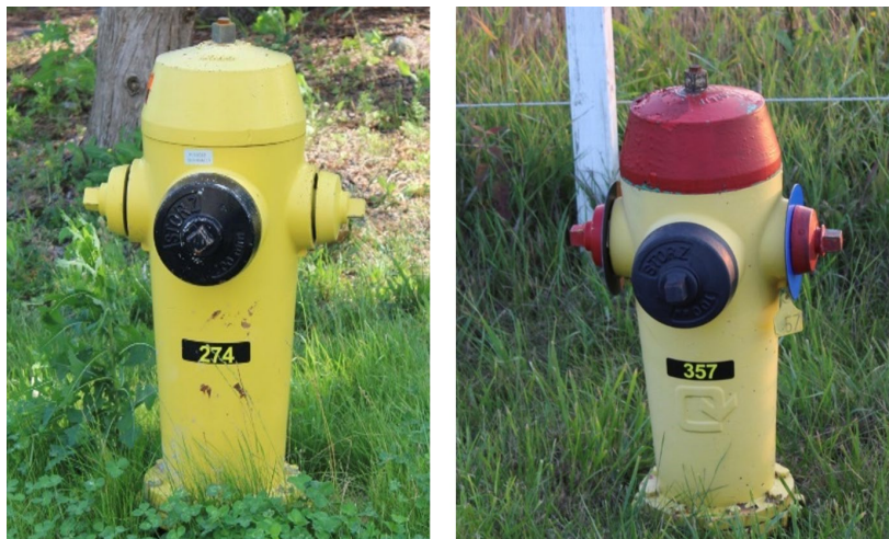
Figure 15. Municipal fire hydrants in Essex.
