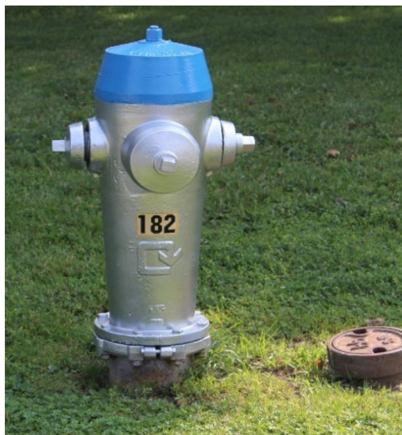
Figure 17. Private fire hydrant in Essex.
